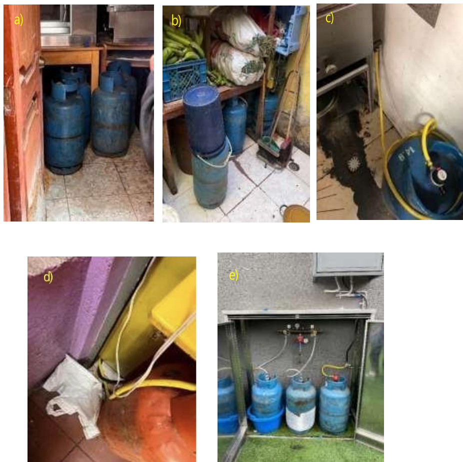
Figure 1. Non-compliances related to LPG cylinders: a) Cylinders surrounded by combustible materials, b) Cylinders located in confined spaces, c) Inadequate connection hoses, d) Electrical wiring and ignition sources around cylinders, and e) Lack of natural vaporization in cylinders.
